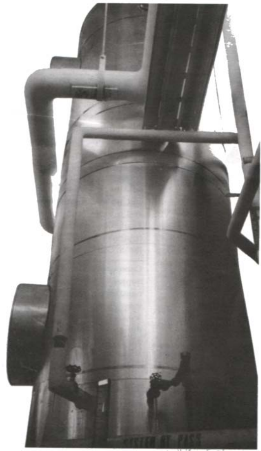
The FLU-ACE® heat recovery system at the St. Vincent Hospital in Ottawa, Canada.
