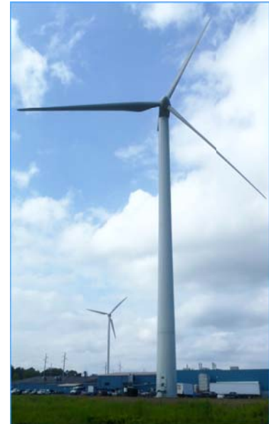
250kW and 850 kW Wind Turbines at HARBEC, Inc.'s Manufacturing Facility in Ontario, NY
